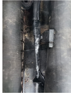
Wiring & vacuum pipe
